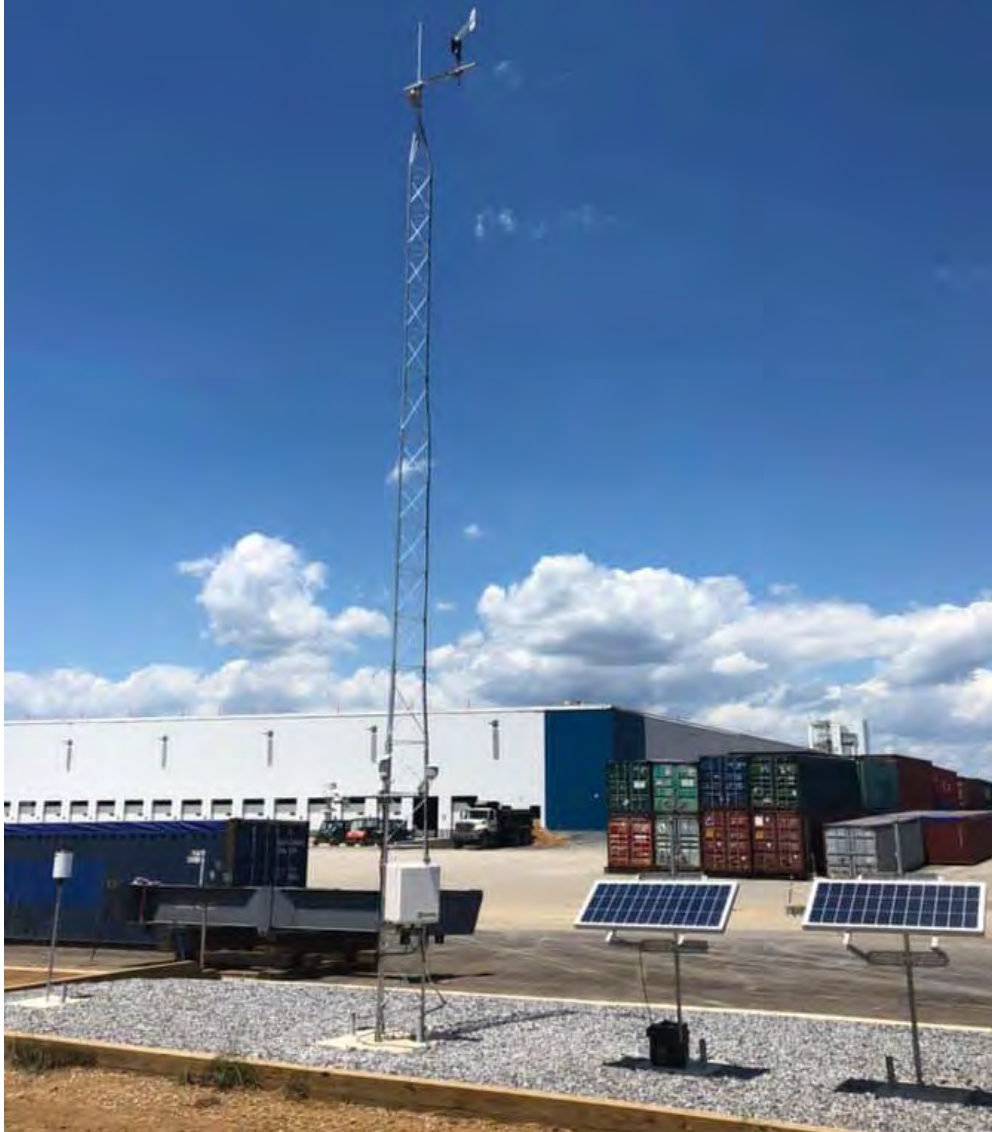
Figure 4: ROCKWOOL Meteorological Monitoring Location
